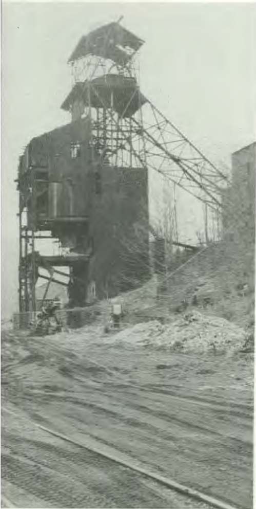
Tipples dump (or "tip") coal from mine cars into trucks or trains. Abandoned tipples, such as this one, pose hazards to people who venture onto them or into the shafts they top.
