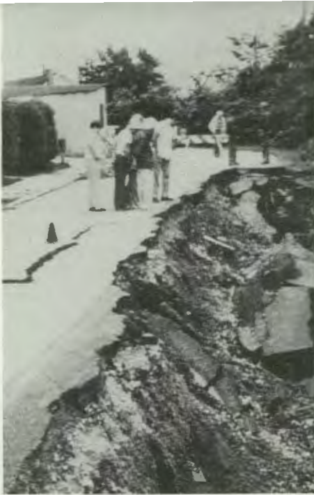
This road was built on mining waste piled alongside a creek. The road collapsed when the creek washed away the base of the pile.
