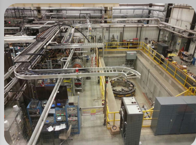
7625 high bay supports Proto-MPEX helicon plasma source and plasma materials interaction R&D
