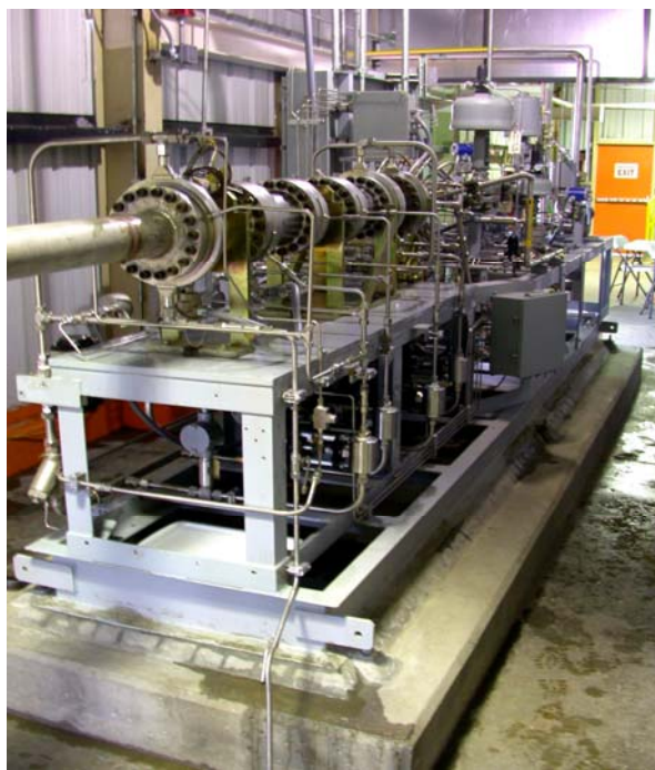
Fig. 5. Fuel-Oxygen Combustor (Courtesy of Clean Energy Systems).
