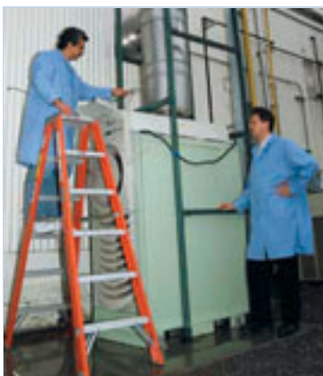
Researchers at the CHP Integration Lab examine a microturbine that provides power.
