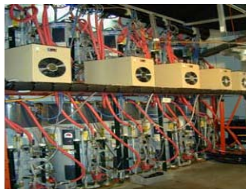
Water Heater Test Facility
